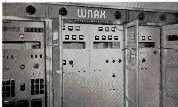
WNAK—YANKTON —On the air since 1926, this South Dakota station recently modernized its broadcast facilities, installing a General Electric 5 kw AM transmitter.
